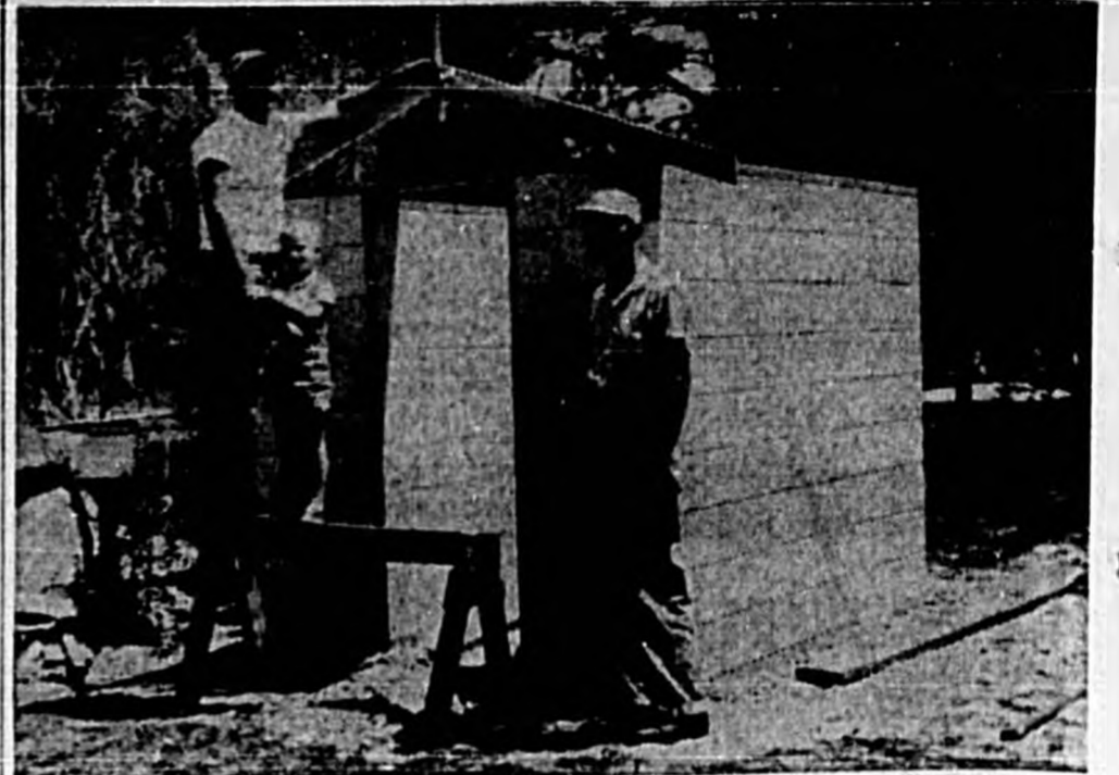
A NEW PUMP HOUSE is under construction at the Enterprise Cemetery and when electricity and the pump are installed, another dream will come true for the community. In the past, all water has come from a centrally located hand pump. A pipe line running the cemetery's full length will be laid and 12 faucets and hose connections will be installed. Shown working on the building is Wilbur Bruce, president of the Cemetery Assn., son, Joe and Sidney Emanuel, association trustees. (Cox Photo)
