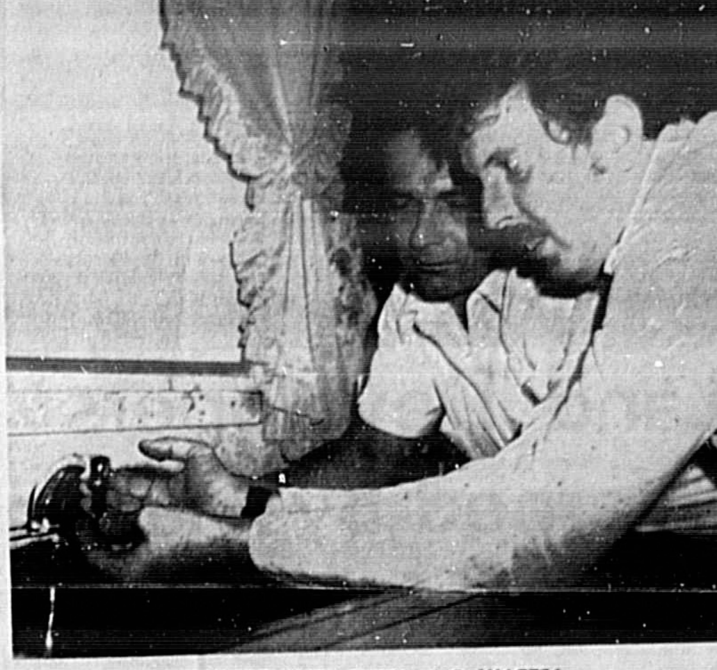
FAUCET WIDE OPEN—NO WATER! Winter Springs residents John Griffiths and Paul Lariviere demonstrate how to install a faucet and meter in the subdivision. Customers of utilities in the subdivision are urged to boil their drinking water. (Ann Riley Photo)
