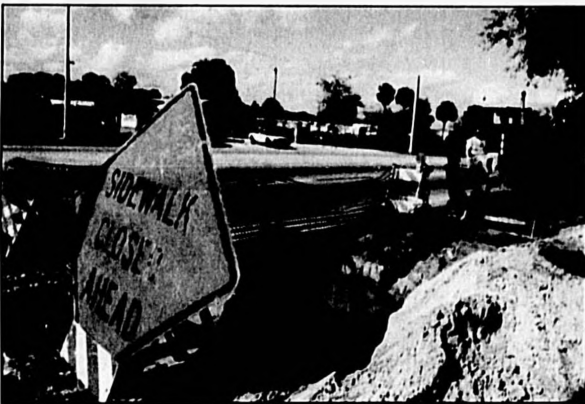
Dan Boomershine, of All-Bore Inc. of Boonville, Ind., uses a machine to bore horizontal holes under the sidewalks and streets along Highway 17/92 in Sanford. The will be used to run conduit for fiber-cable for tele-phones and high-speed data transmissions.
