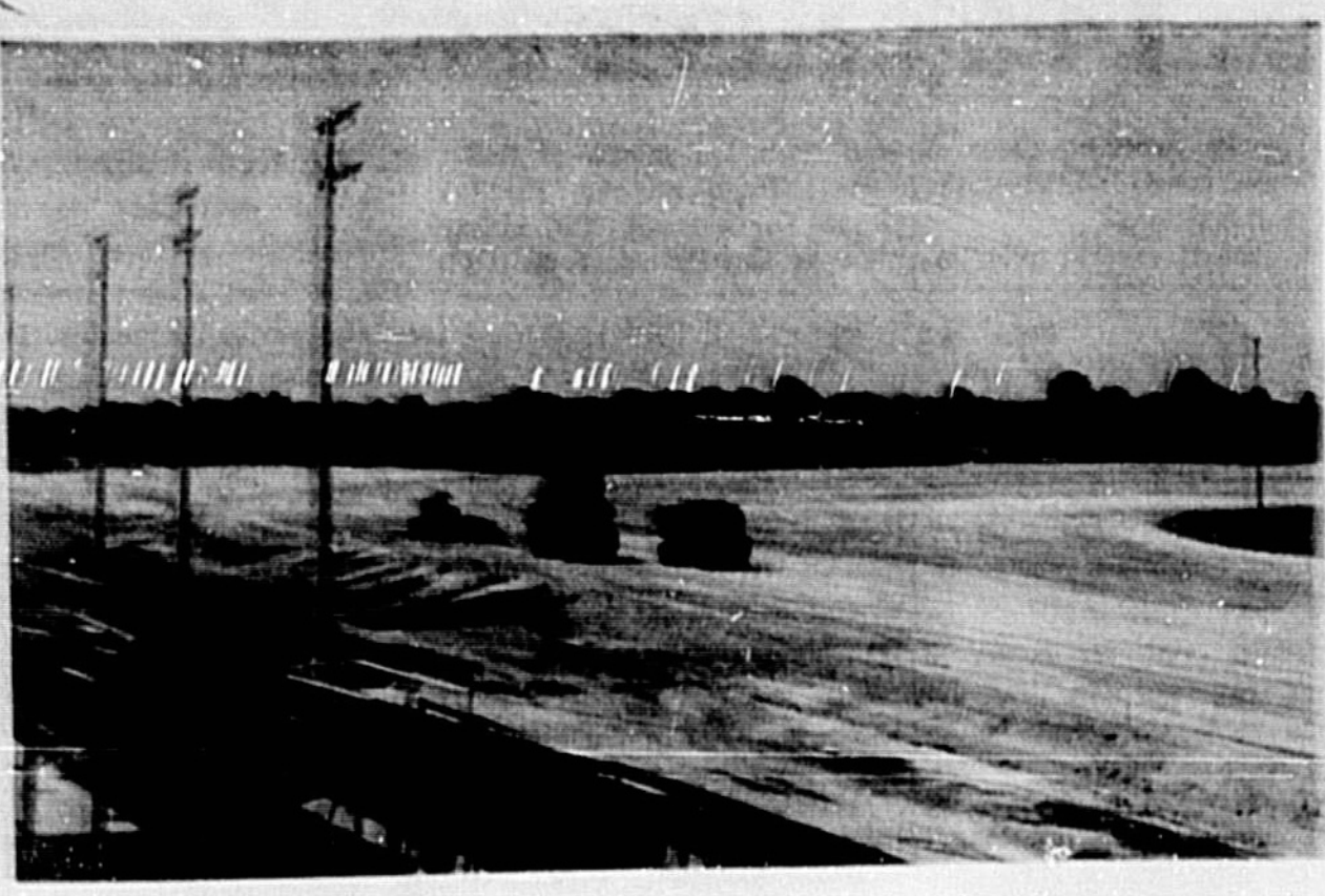
A NEW three-quarter mile race track is being constructed at Seminole Turf Club in Casselberry in anticipation of the opening of a thoroughbred racing season on April 17, 1970. Approximately 2,500 yards of clay are being hauled in daily to build the new course. The parking area is being expanded and work is expected to begin Monday on the 12,000 sq. ft. two-story club house to be built on the south side of the present grandstand. (Jane Casselberry Photo)
