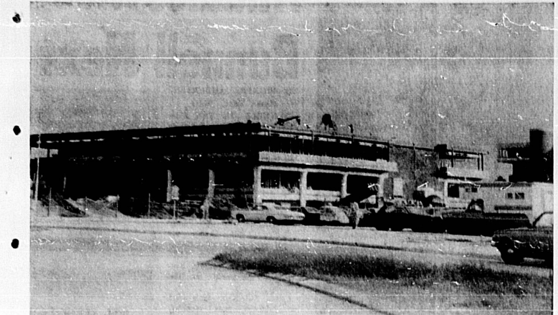
A NEW 5 story administration building, being built at Florida Technological University at a cost of $2.2 million, is scheduled for completion in April and will house offices for administration, faculty, and student government as well as classrooms. (Jane Casselberry Photo)
