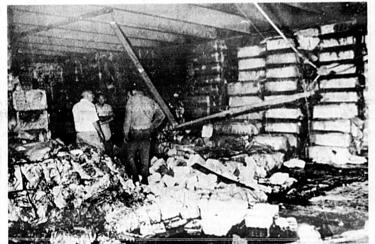
REMAINS OF DAMAGED STORAGE AREA Officials and sheriff's investigators probe fire scene
