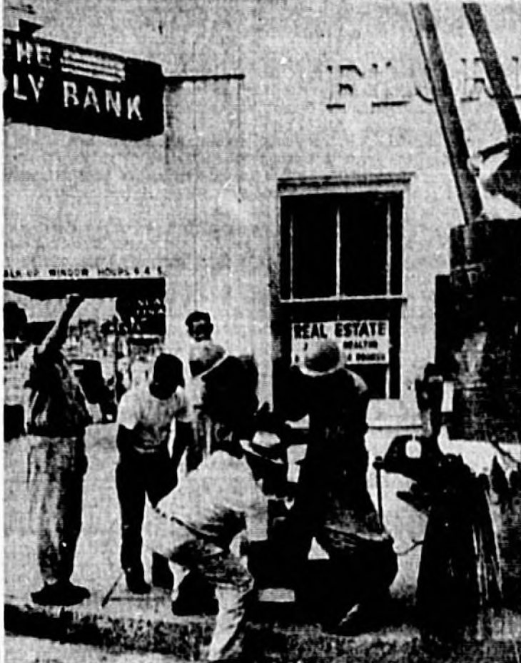
BRIGHTER CITY—Workers were busy installing the new lights this morning at the Park Ave.-First St. intersection. The new feature will put out 20,000 lumens of light to add to the brightness of the Sanford downtown section. (Photo by Jameson Studio)
