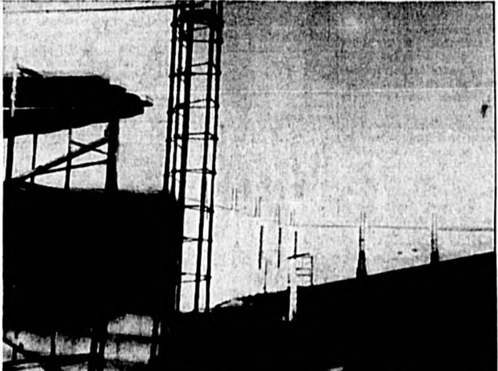
CONSTRUCTION IS PROGRESSING on the new $700,000 Cinema Theater in Seminole Plaza at Casselberry with the opening scheduled for Christmas Day. The Cinema will seat 900 persons and will be the county's first indoor theater outside of Sanford. (Herald Photo)
