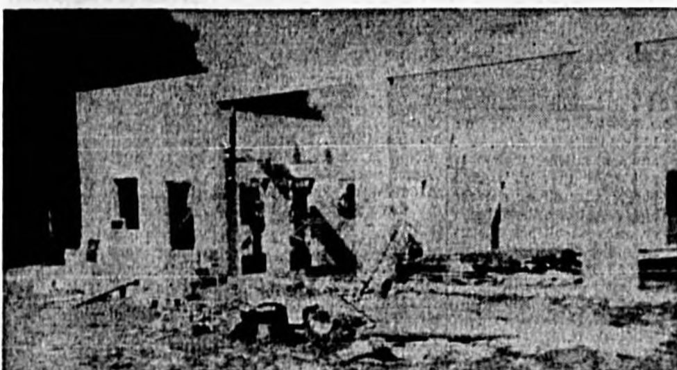
A NEW FIRE STATION, under construction by the Lockhart Volunteer Fire Dept. which serves the Bear Lake area of South Seminole County, is shown in the above photograph. The department's latest successful money raising project was a comedy play, "Womanless Wedding," presented twice last weekend to raise funds to roof the building. (Herald Photo)
