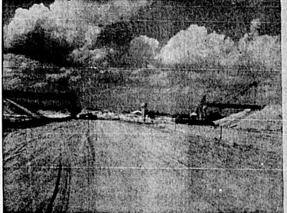
. . . and this will be the cross-over at Lake Mary Boulevard. County Commission is endeavoring to have the State Road Department and federal government to place a cloverleaf here . . . .
