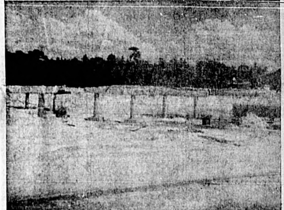
. . . while presently traffic is being routed around this bridge construction over Highway 434 at Sandlands Springs. However, it is only a brief detour and . . . .
