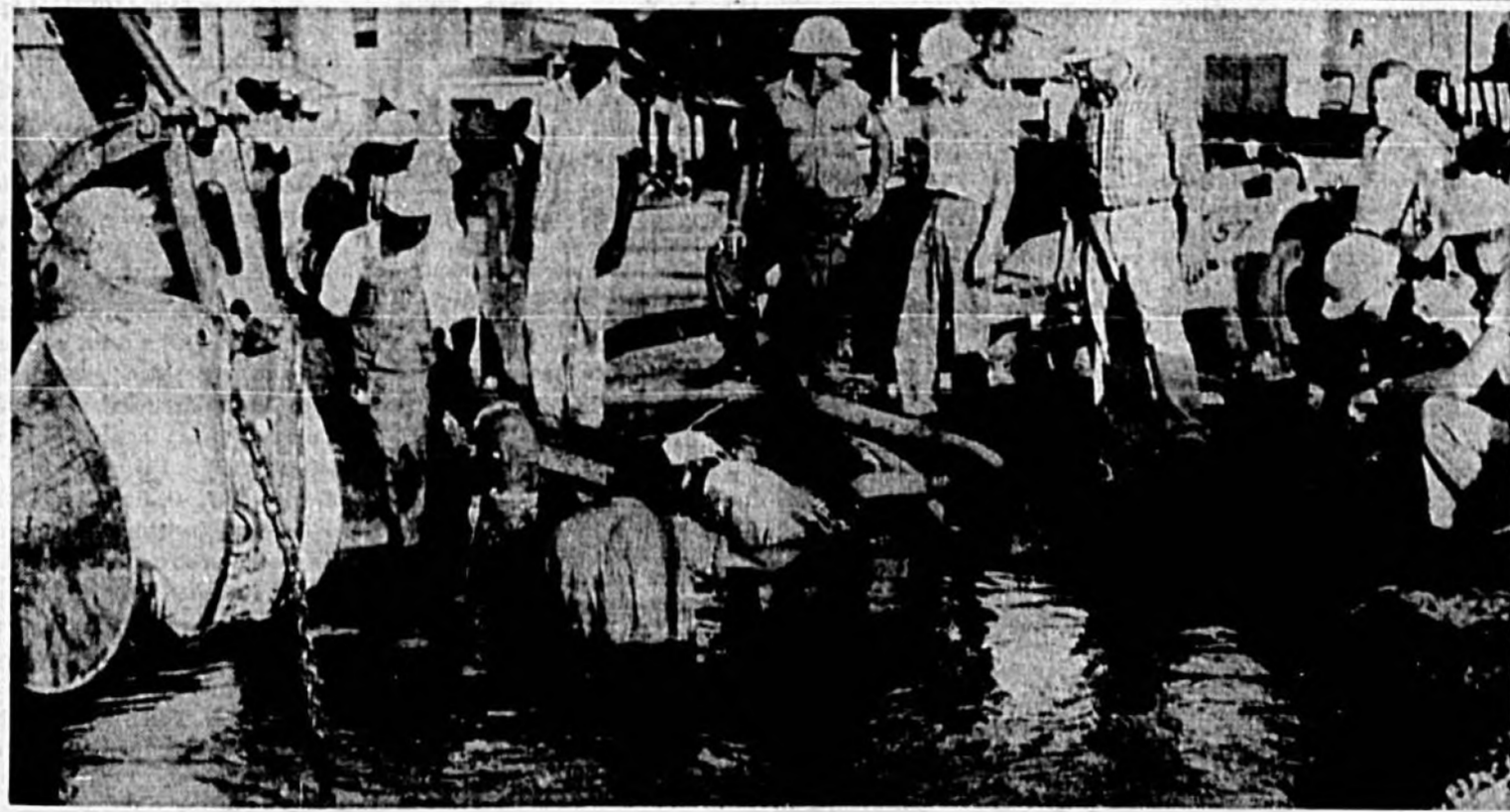
City Crews Work Frantically To Plug Up Broken Water Main (Herald Photo)
