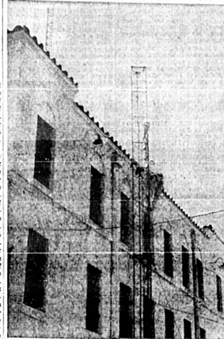
A 150 FOOT TOWER goes up at the Seminole County Jail as a workman attaches the third section of the nine-section steel spire. The tower is part of new radio equipment recently purchased by Seminole County Sheriff J. L. Hobby that will tie in with the Civil Defense system. (Staff Photo)
