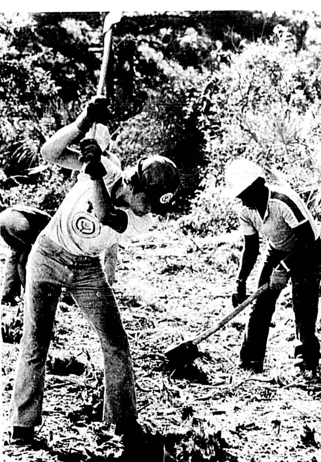
Blair Davison (foreground) removes Palmetto roots from new parking area at Nature Center.
