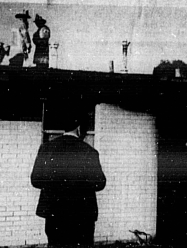
FIREMEN CHECK FIRE DAMAGE Seminole County firemen check roof for damage after dousing flames Wednesday afternoon at 2807 Truman Boulevard Lincoln Heights, home of Mary Stevens. Fire was believed to be caused by a can of gas in a storage area and firemen reported approximately $5,000 damage. (Herald Photo by Bill Vincent)
