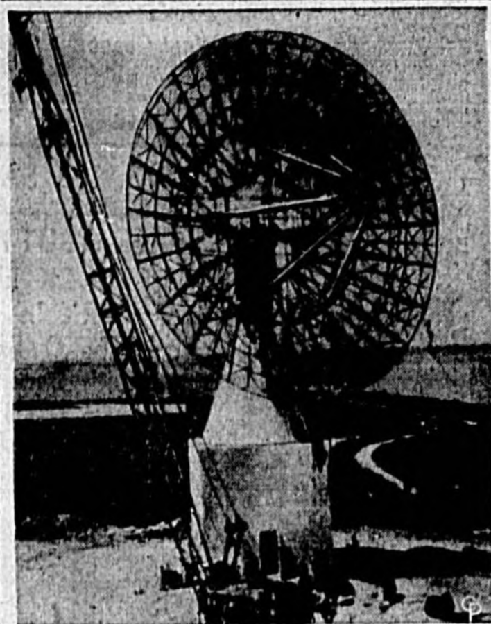
WILL TRACK U. S. SATELLITE—Workers rush to completion at Cape Canaveral, Fla., one of the five radar antennas being erected to track the U. S. test satellite scheduled for launching next month. Each will have a range of 1,000 miles. They are being placed on a 5,000-mile route stretching from Florida to the Ascension Islands.
