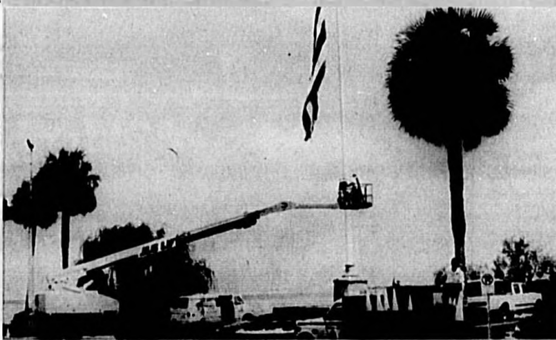
Steve Wallace, of Wallace Welding, works in a bucket at the flag pole in Sanford's Memorial Park on the lakeshore. M&M Flags and Banners, in Casselberry, has been contracted by the city to repair the flag after it has been lowered. The flag was damaged by the winds of Hurricane Erin, but could not be taken down because of halyard problems.
