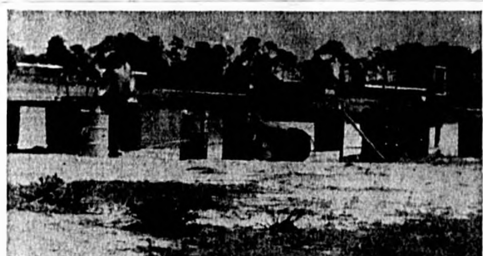
CHULUOTA'S BEACH on Lake Catherine is under repair and a number of additions are being made in preparation for the busy summer ahead. The above photograph shows a new lifeguard stand, at right, built by Bill Lampinen and N. E. Runyon and Charles Bell are shown, at left, painting the raft and lifeline drums. (Jones Photo)
