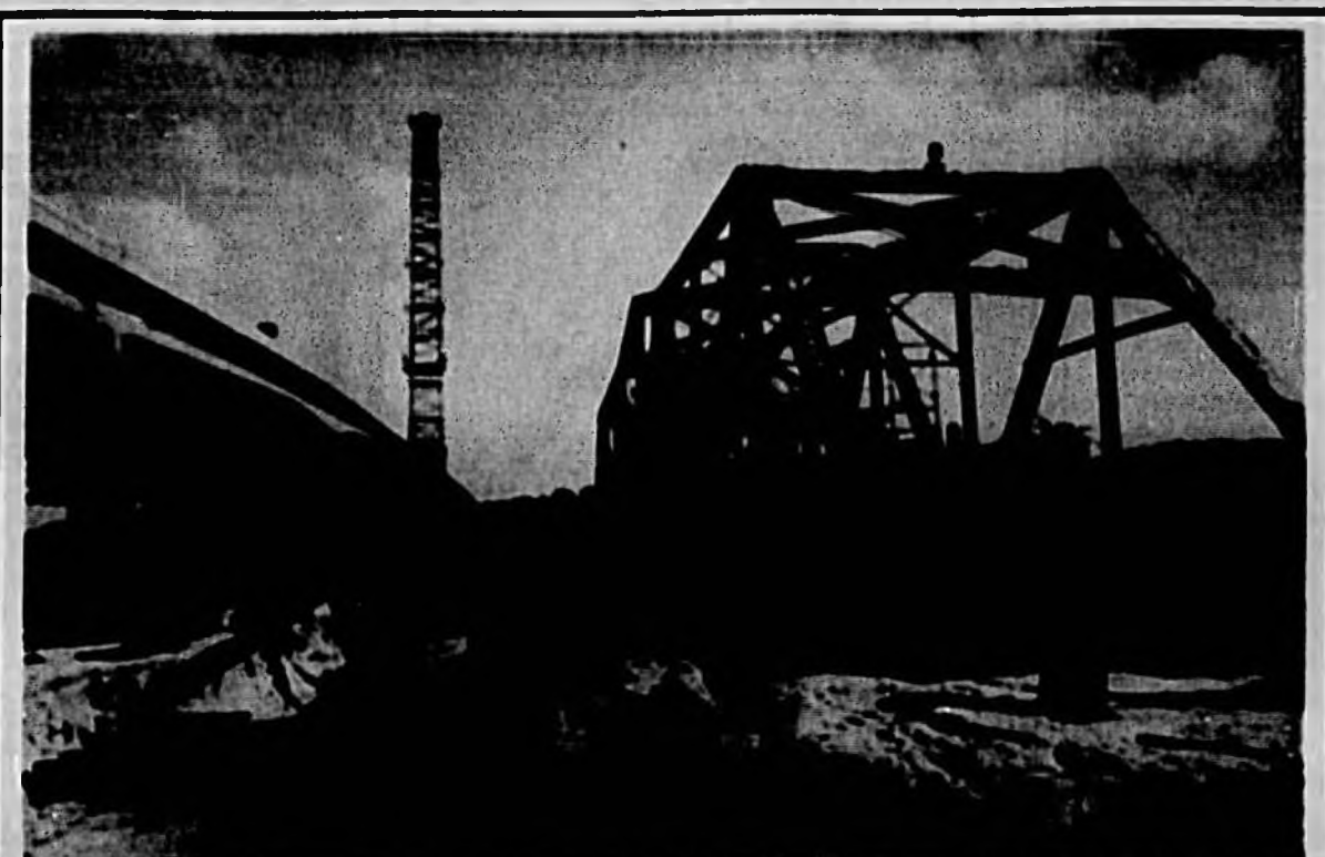
Out with the old... Work continues to turn the 57-year-old U.S. Highway 17-92 bridge over the St. Johns River into a fishing pier. Last week, the old iron and wood structure was carefully moved from its historical resting place to its final spot nearby. The bridge's new replacement stands nearby.
