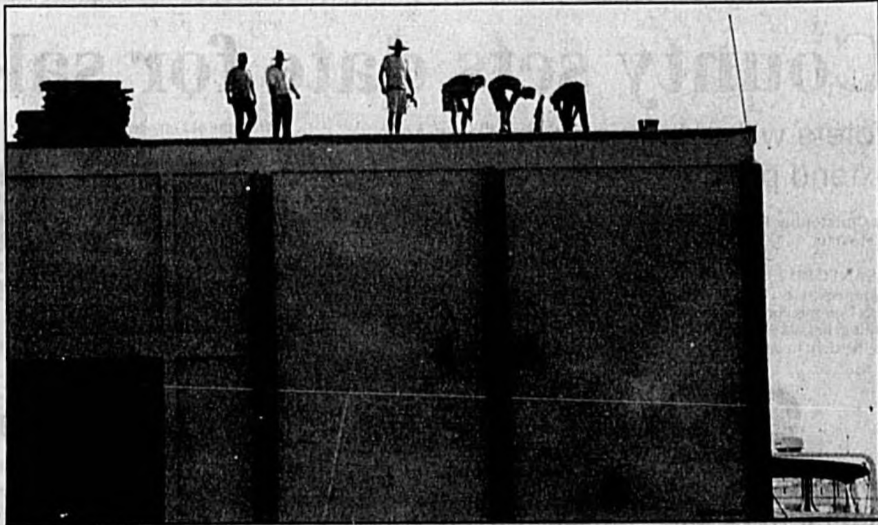
Workers from Adcock Roofing Co. of Sanford begin work on replacing the roof on the Monroe Marina Harbour building. The roof was damaged a few weeks ago during a rough storm that brought heavy winds and rain.
