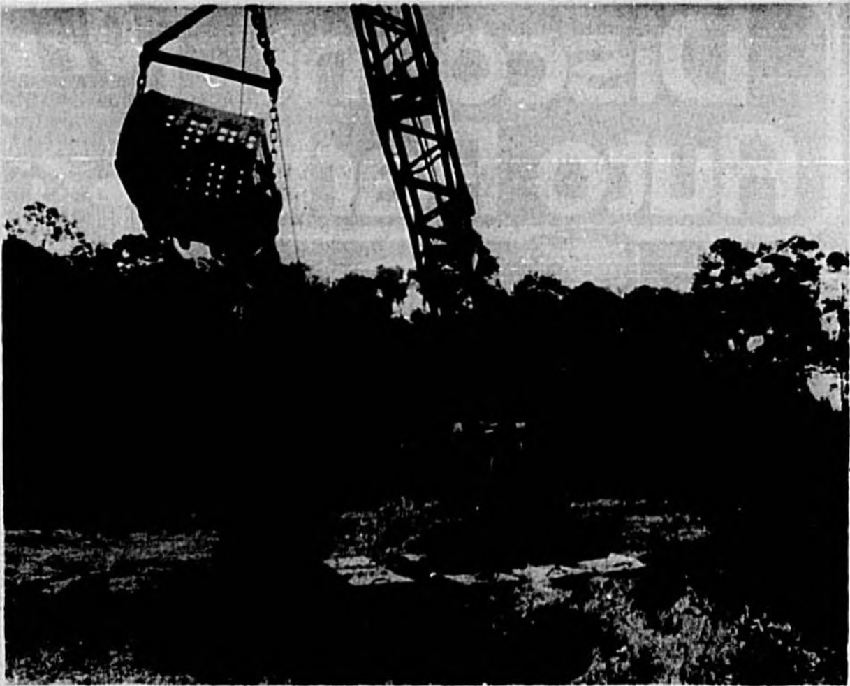
A dragline operator at Lake Gem maneuvers a large mat to place in front of the dragline to keep it from sinking. Cleanup of the city park has been sought for years.
