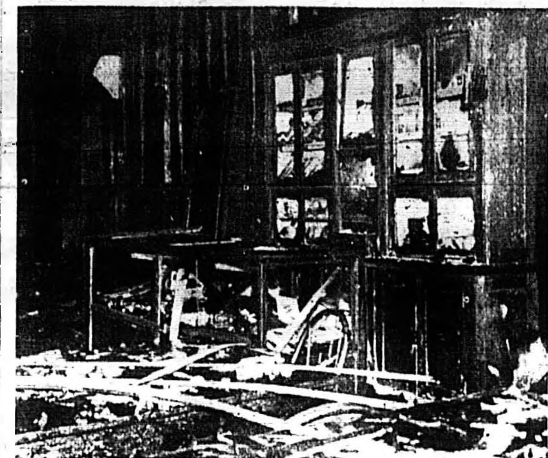
DEBRIS is scattered through the lobby of the old Canfield Hotel in damage from fire which started in the lobby. The fire started in the lobby and spread rapidly through the building and its six-story annex.
