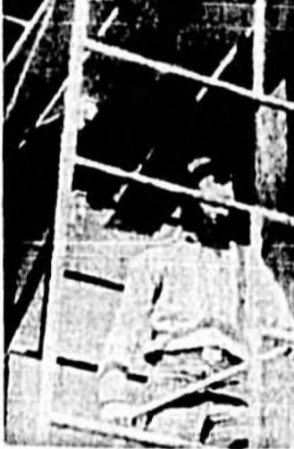
SAILORS FROM VAH-1 pitch in to aid in the project of improvements at the Sarepta Rest Home. Here, D. C. Plumley and D. A. Desbroids are shown climbing the scaffold to brush off loose paint. Other men working on the ground included P. V. Shelley, R. O. Wilson, L. W. Kivel, D. N. Coles, J. L. Drugach and W. C. Wooten.
