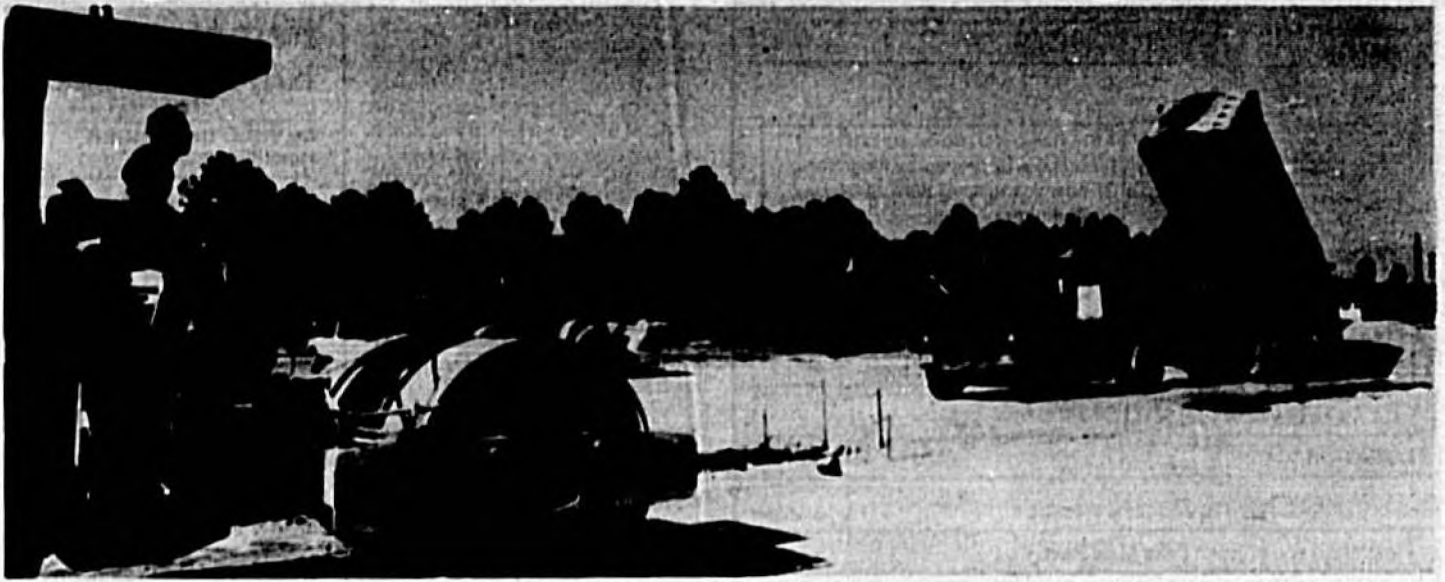
A shopping center will open later this year on this site off U.S. 17-92 near Seminole Community College.
