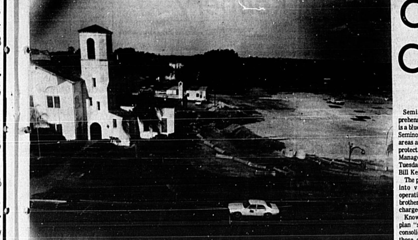
NEW SANFORD CITY HALL SITE Construction workers of Williams Development Co. prepare to re-route storm sewer lines on the construction site of Sanford's new $14 million city hall. When the new building is completed next January, the workers will demolish the current city hall, which is 50 years old. Work began on the new structure March 29. Funds for the project were provided by the U.S. Commerce Department's Economic Development Administration.
