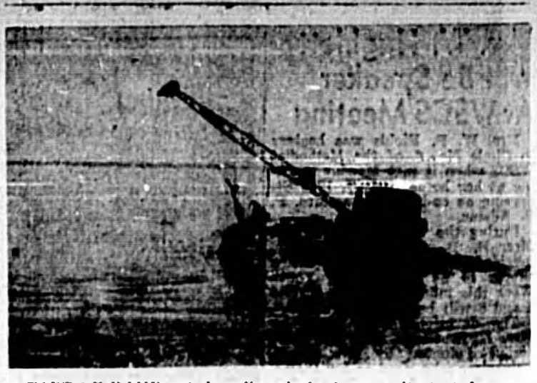
START OF RAMP —A drag line rig is shown as it started scooping a trench in the bottom of Lake Douss in which to lay an outfall pipe for the City sewer and water program, using the reidue to build its own ramp out into the lake. One drag line rig broke down about 500 feet out in the lake and was replaced. Work on the outfall pipe and interceptor main is being done by Hamby and Simpson, Orlando. Superintendents of the project are Oliver and James Dinmore, brothers. (Photo by Warren Knowles, City manager)
