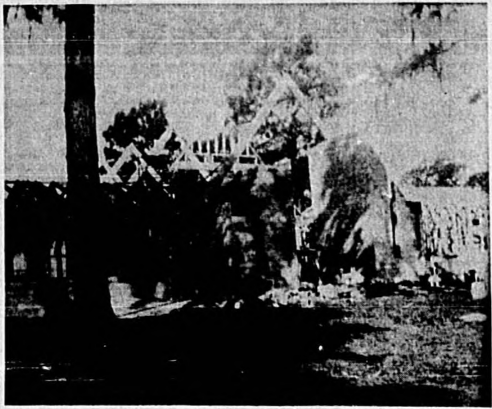
THE ARCHITECTURAL beauty of the new Ascension Lutheran Church is becoming apparent to those passing through Casselberry. Pastor C. R. Zehnder has set June 3 as a tentative date for laying the cornerstone in the new church which is expected to be completed within the next two months. (Herald Photo)
