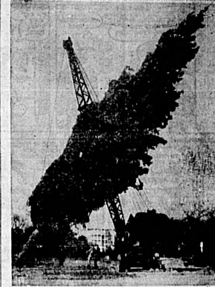
A CRANE LIFTS this huge Engelmann spruce on the south lawn of the White House as the nation's capital takes on a Christmas glow. The tree, to be lighted by President Eisenhower on Dec. 20, will be focal point of the world-wide peace pageant. The President will broadcast an around-the-world message. (International Soundphoto)
